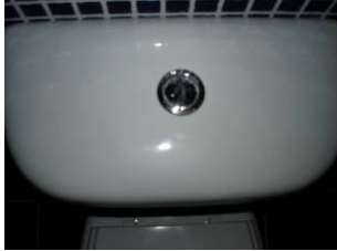
Figure 5.6: Double flush toilets
