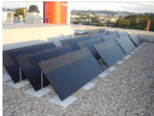
Figure 5.10: Solar collectors in the roof
