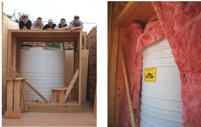
Figure 9a/9b. Hot water storage tank with insulation.
