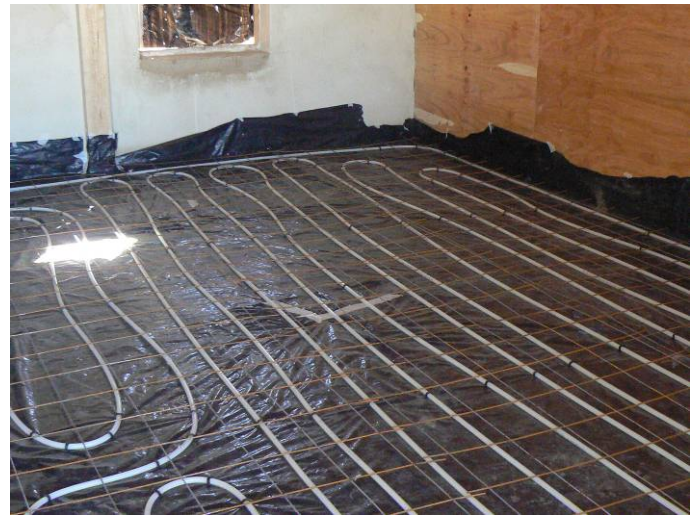
Figure 10. Plastic pipes for under floor heating.
